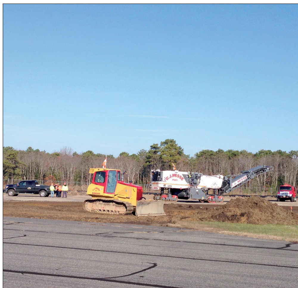
The Federal Aviation Administration Technology Research and Development Team will use a decommissioned taxiway at the Cape May County Airport as a research test bed for airport-safety initiatives.
