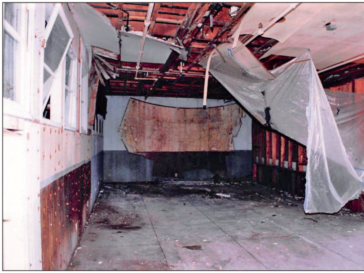
A room on the north side second floor shows water damage. This is a result of the deteriorated roof above, which will be repaired through grant funding.
