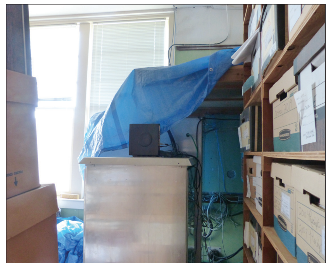
Jack Fichter/CAPE MAY STAR AND WAVE A tarp covers a radio equipment cabinet in a second-floor records room at the Cape May police station to prevent water intrusion.
