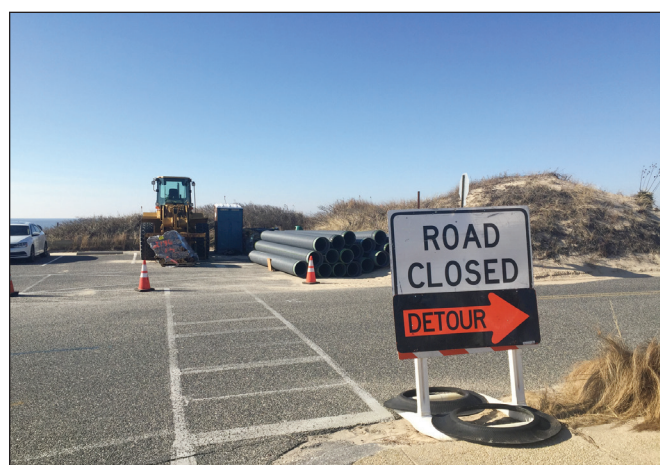
Asphalt Paving Systems has begun work on the Beach Drive Pedestrian Safety and Road Improvement Project.
