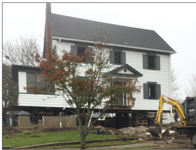
Jack Fichter/CAPE MAY STAR AND WAVE 901 Benton Ave., a contributing home to the Cape May Historic District, before construction began.
