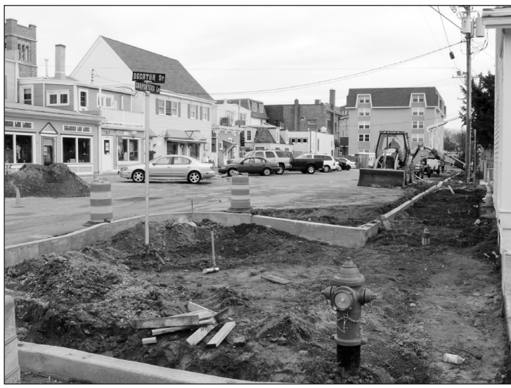
Above, construction on the south side of Carpenters Lane at the intersection of Decatur Street began last week in order to make ADA improvements.
