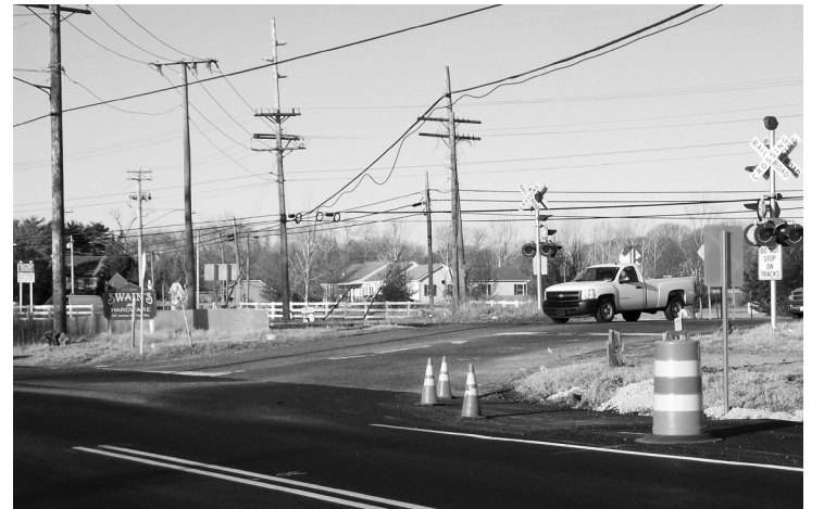
Christopher South/Cape May Star and Wave Top, construction on the extension of Breakwater Road. Above, Bennett's Crossing, which will be eliminated at the end of the project.
